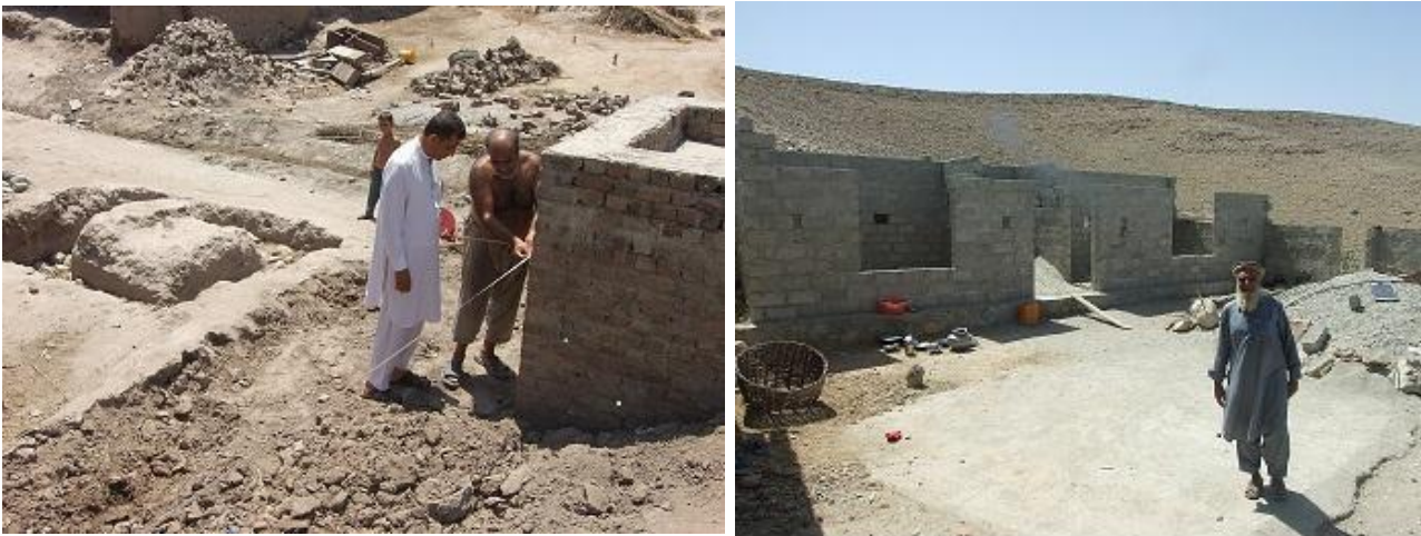
Plotting maps on the ground and field Engineer advice the beneficiary for construction of Shelte
