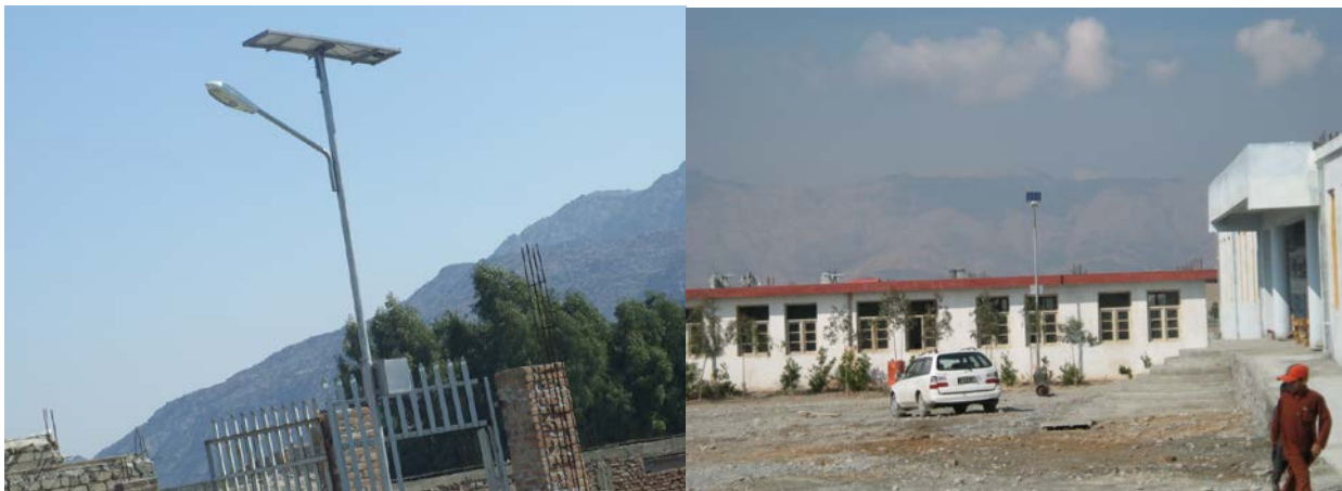
Solar lights installed in Public Area
